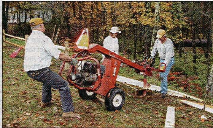
Woody and Christine Fogg help to guide the posthole digger as Ken Knowlton drills the hole for a fence Thursday at the new Penstock Park in Belmont.
