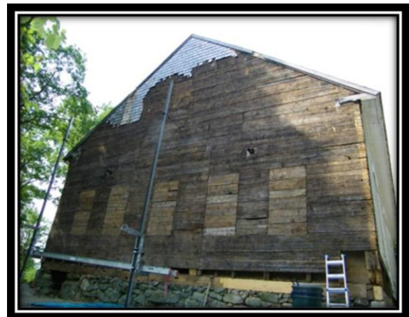
After the east-end shingles were removed, original window locations were revealed at the Province Road Meeting House.
