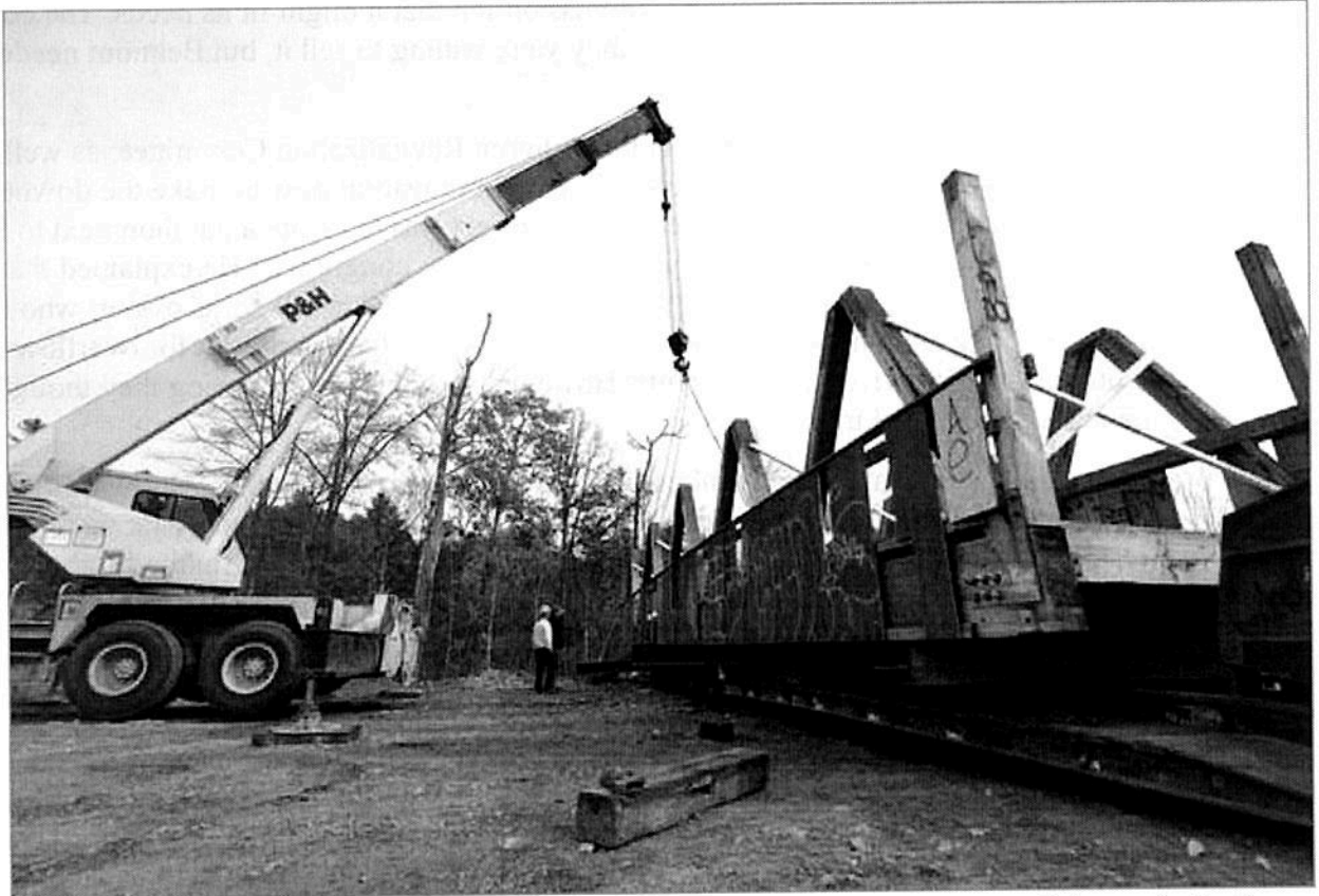
A COVERED bridge from Dover was recently moved to Belmont as part of the revitalization plan in Belmont Village. Crews are seen here off loading the last section of the bridge Wednesday.
