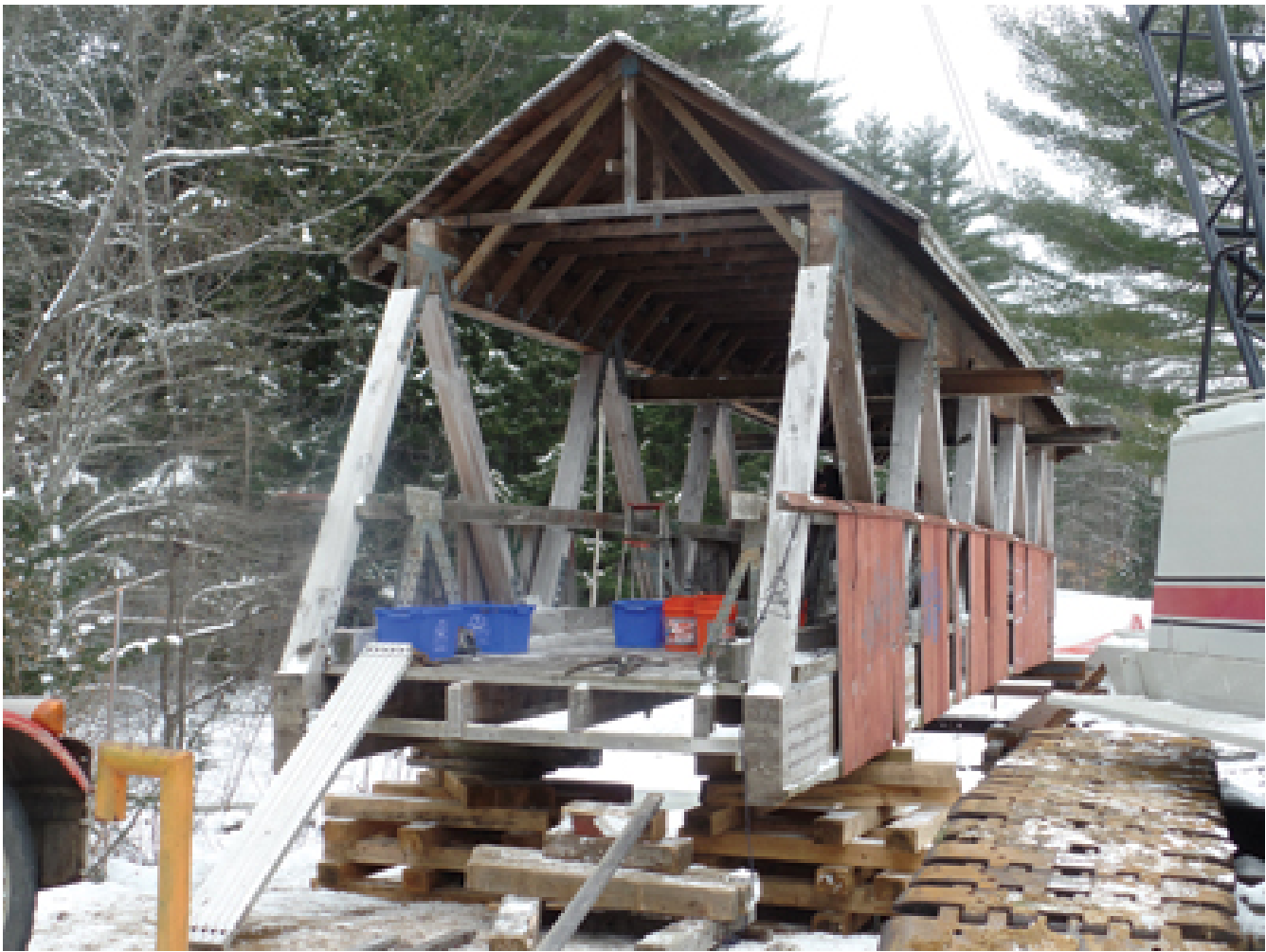
1st section set on beams, with roof being lifted in place with LE Roberts' 75 ton crane (Norm Jackson)
