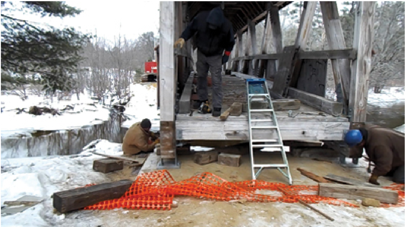
Woody Fogg (left), Ken Knowlton (on bridge) and Jeff Roberts (right) guiding bridge on to bearing pads. (Rick Ball)
