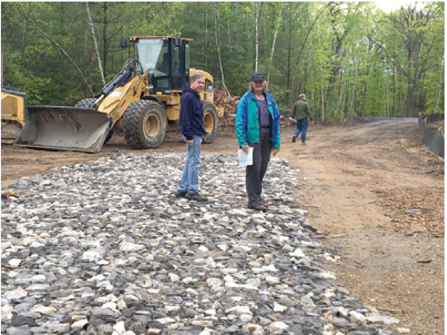
Donna Hepp and an unidentified man walk near the beginning of the Winnisquam Scenic Trail which is under construction. The town expects the project to be completed by mid summer. (Gail Ober photo/Laconia Daily Sun)
